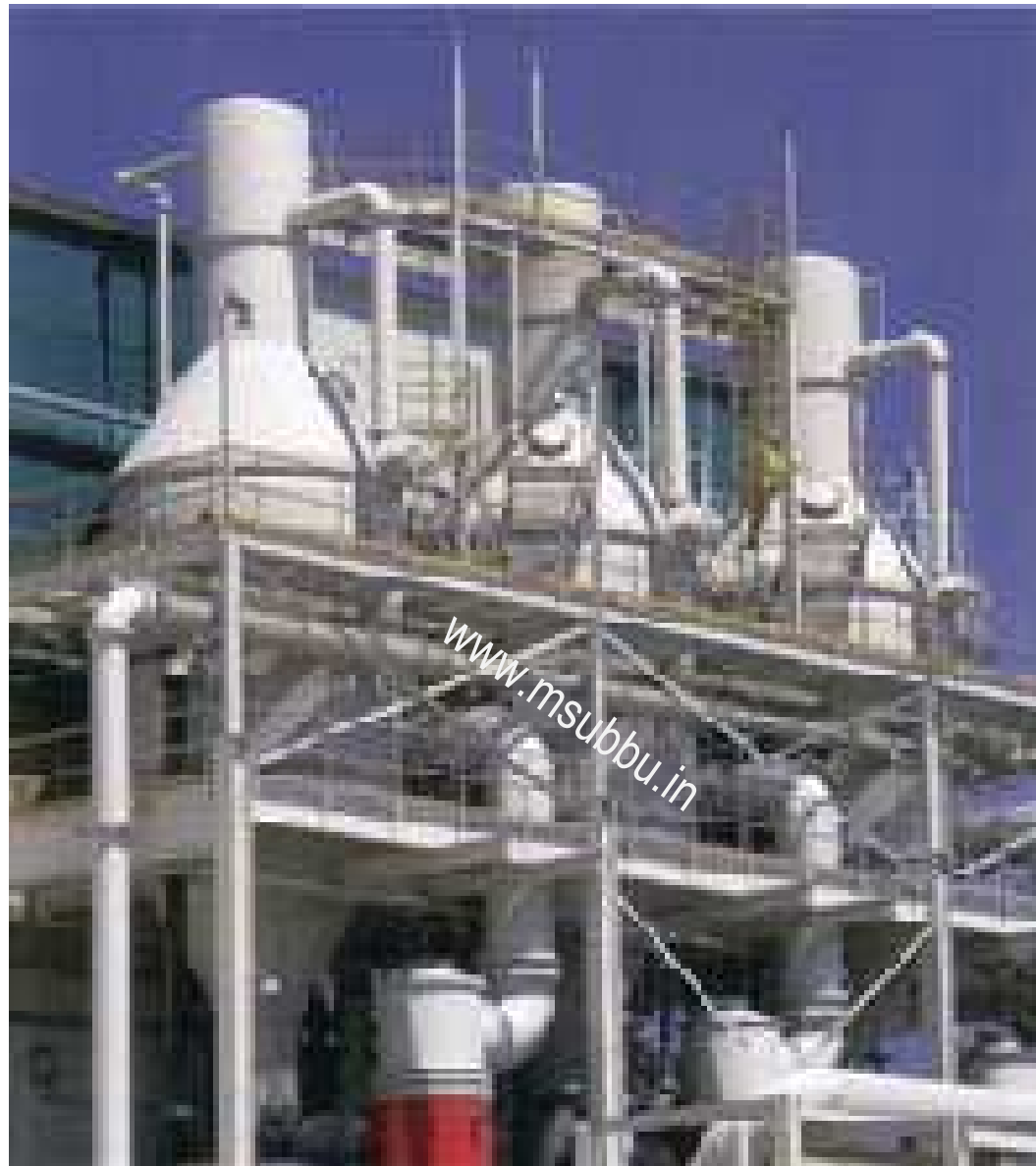
Three-stage, Forced-Circulation Evaporator used to concentrate wet process phosphoric acid
